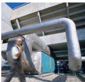
Air handling unit
